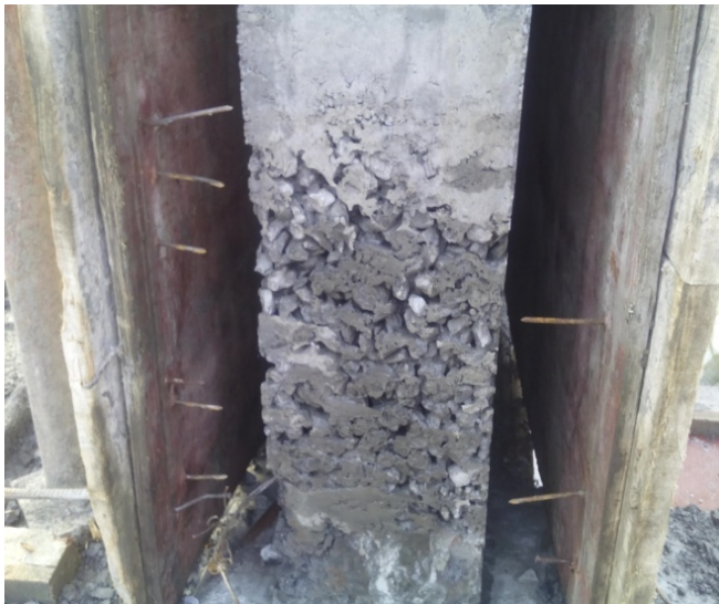
Fig. 3 Quality control inspection report, found concreting
