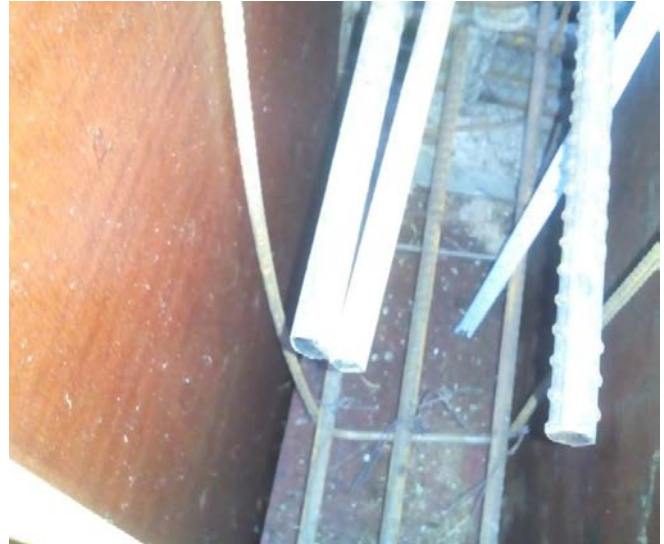
Fig. 1 Quality control inspection report, found inadequate anchorage length and lack of bends 8
