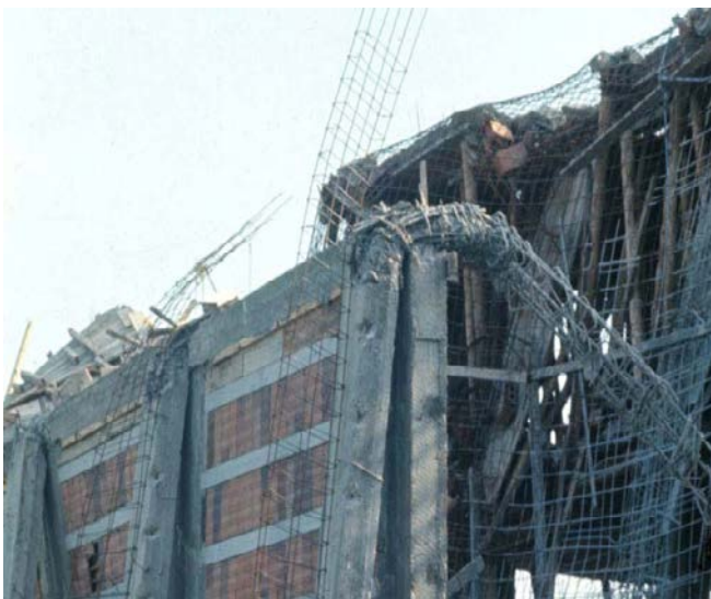
Fig 8 Failure of under construction structure due to insufficient props.
