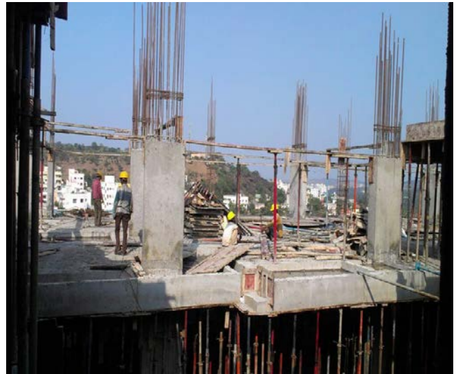
Fig. 9 Quality control inspection report, Cloth wrapping is not done for curing
