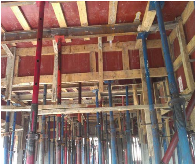
Fig. 7 Quality control inspection report, extra gap found in props than desire and props are not interconnected.
