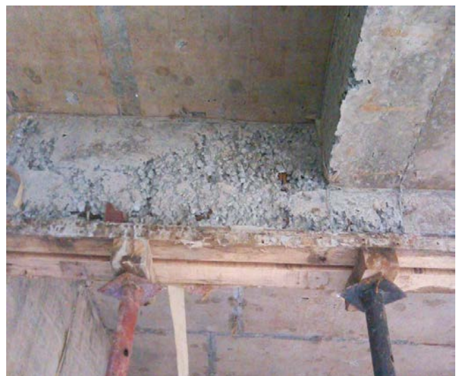
Fig. 6 Quality control inspection report found Honeycomb concreting in beam
