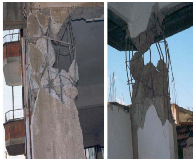
Fig. 10 Failure due to wide spacing of lateral ties as well as low quality of concrete
