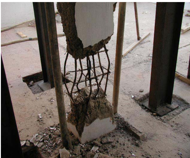
Fig. 4 Failure due to poor quality of concrete
