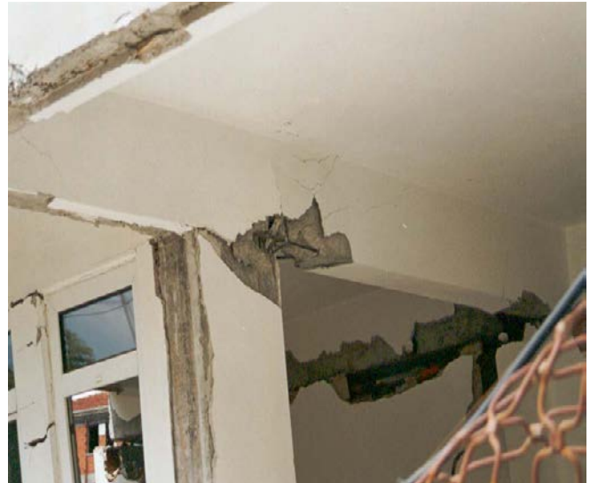
Fig. 5 Failure caused due to porous concrete and rusting of reinforcing bars
