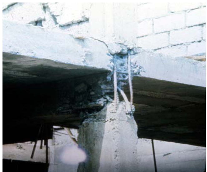
Fig. 2 Failure due to Inadequate Anchorage to reinforcing bars 5
