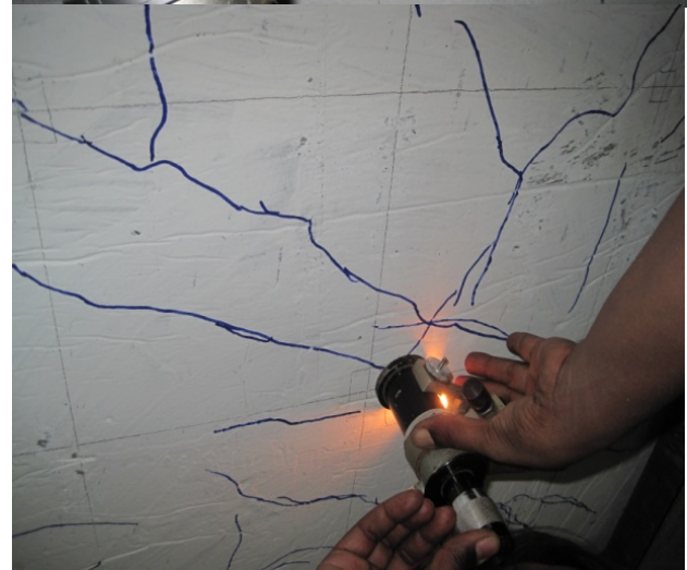
Crack pattern can appear during testing of slab can be seen by using microscope
