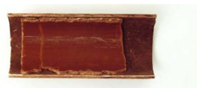
Fig.6. Pipe Cutaway with Calcium Carbonate is Deposited
