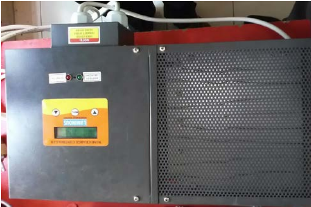
Fig. 3.3 Picture of Charge Controller
