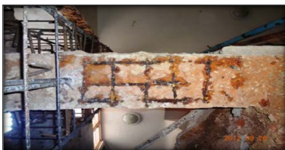
Fig. 2: Severe corrosion on grade beam reinforcement.
