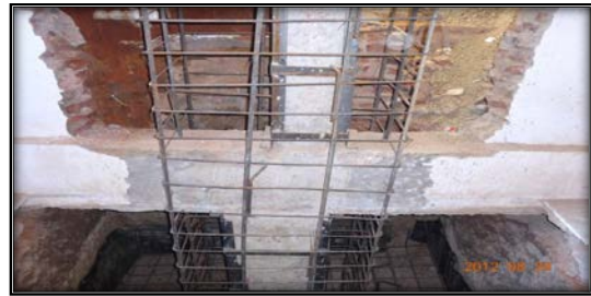
Fig. 3: Severe corrosion on steel bars of eccentrically loaded columns.
