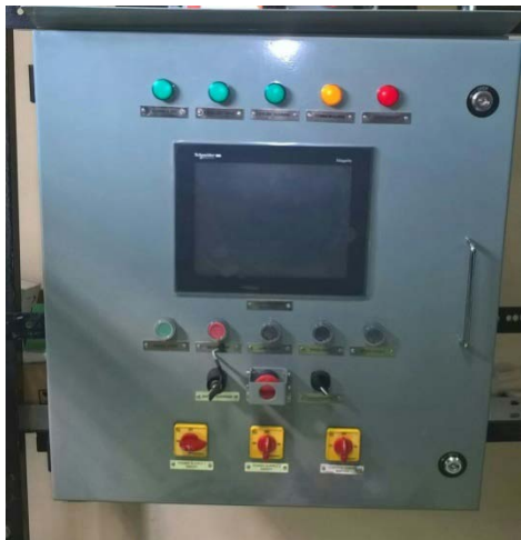
Fig. 4.2 Simulator for control panel
